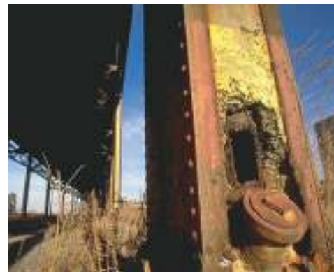
▲ The steel support column of this bridge has corroded because the iron has been oxidized by moist air, yielding \text{Fe}_2\text{O}_3 \cdot \text{H}_2\text{O} (rust).
